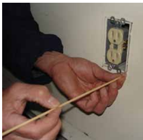
Checking for outside wall insulation behind an electrical outlet with a bamboo skewer.
