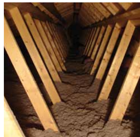
An attic full of Cel-Pak recycled cellulose insulation—locally manufactured.
