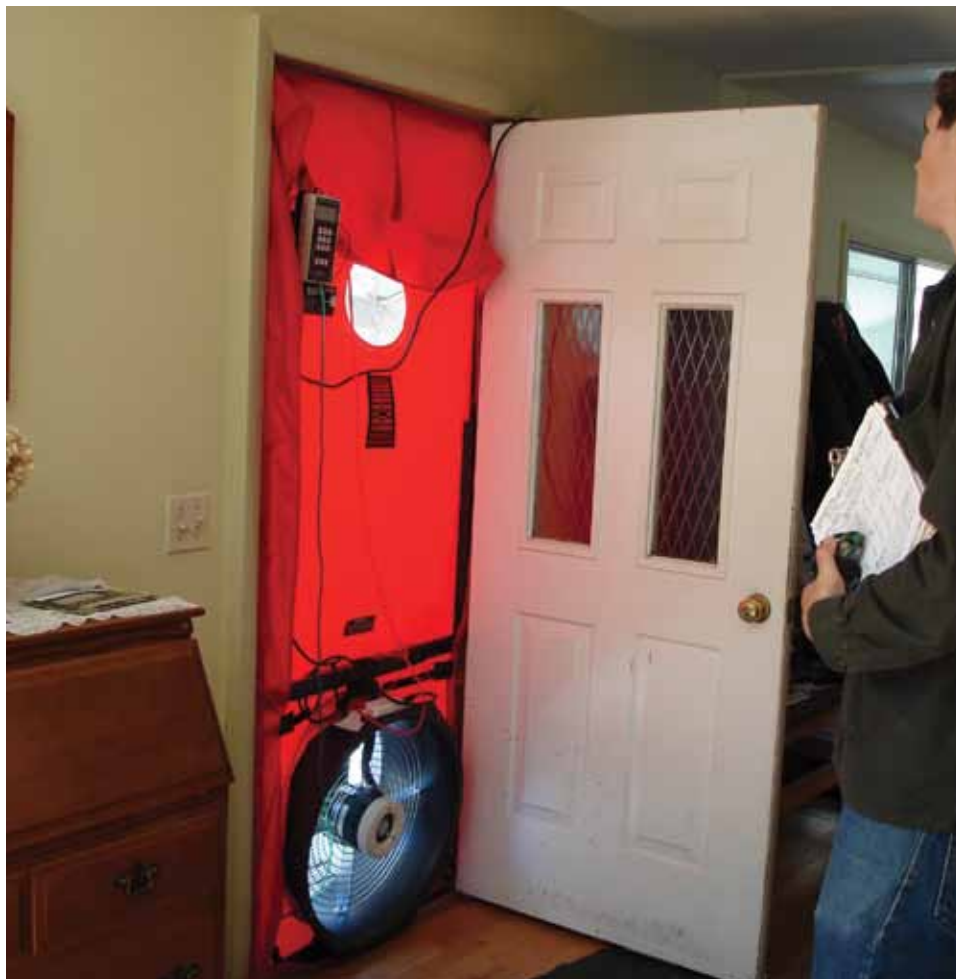
Setting up the blower door to measure airflow and find leaks in the house before sealing.
