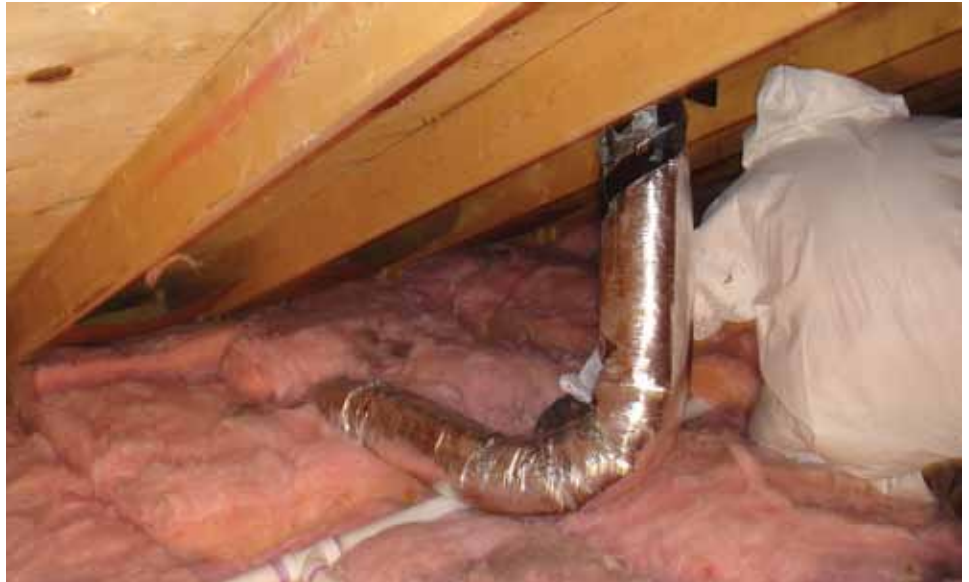
It took two people three hours to seal the gaps in the attic.
